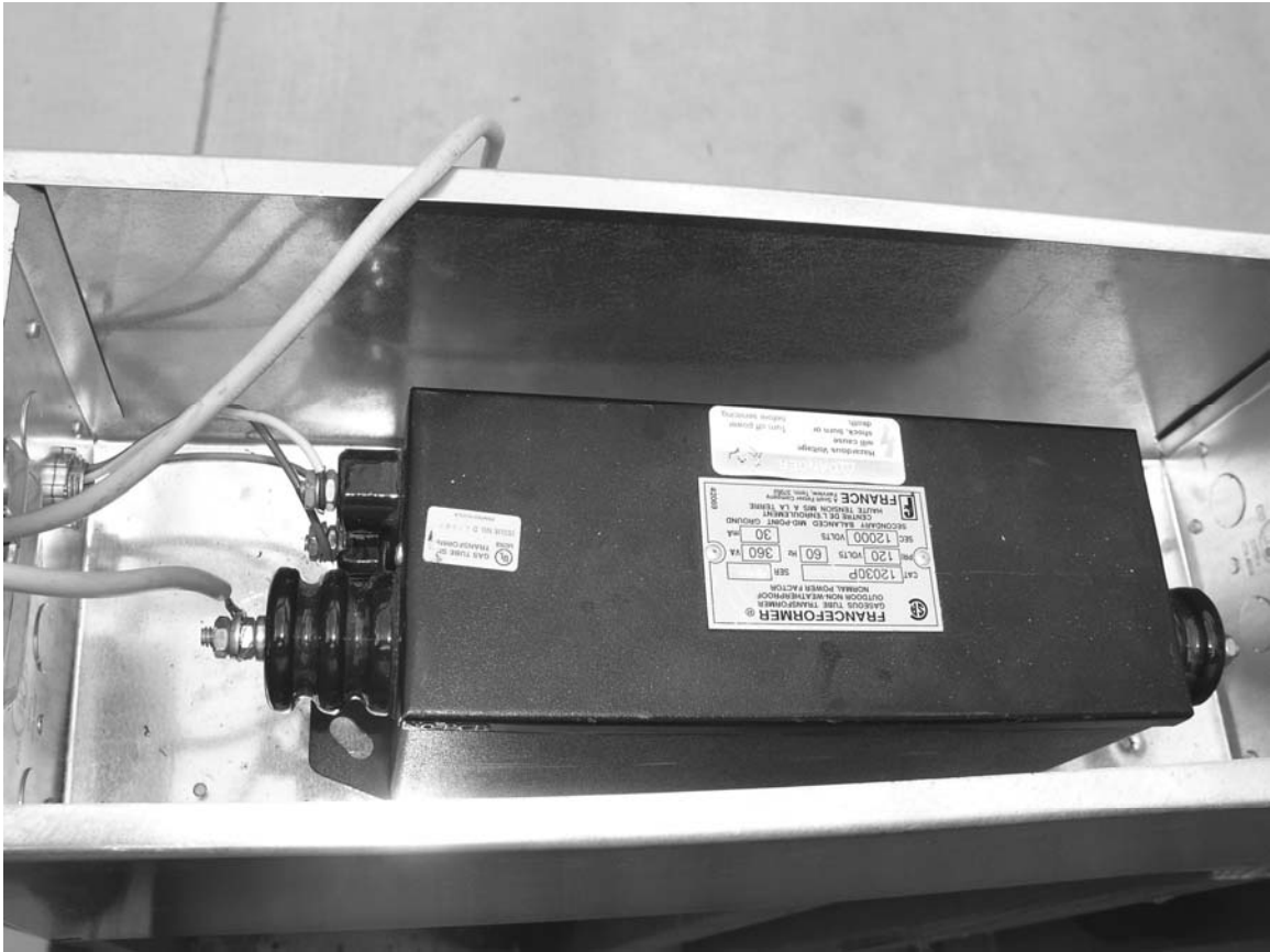
Figure 6 - Non-self contained neon transformer in metal box
