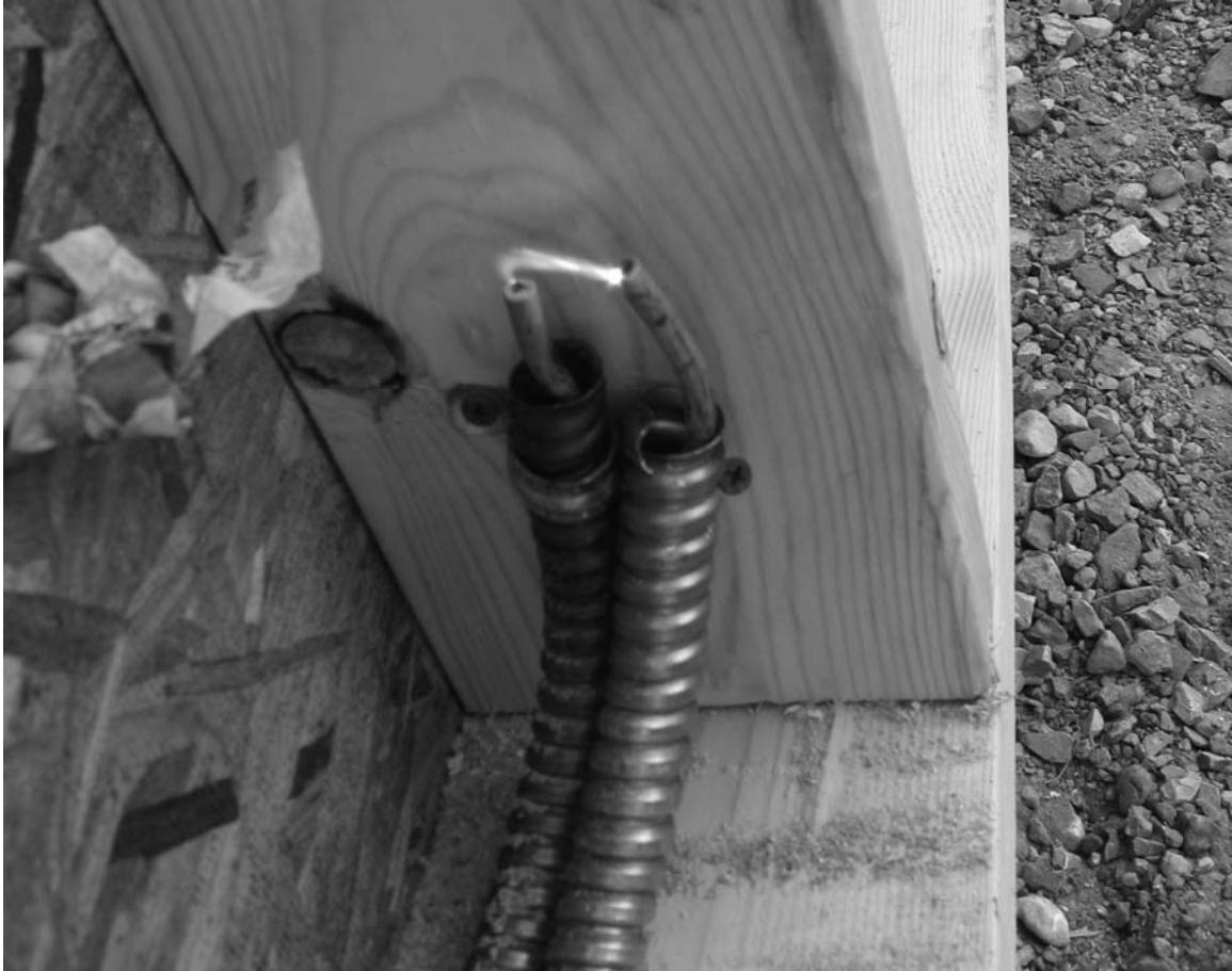
Figure 7 - Three quarter inch long arc from a 12,000 volt neon transformer
