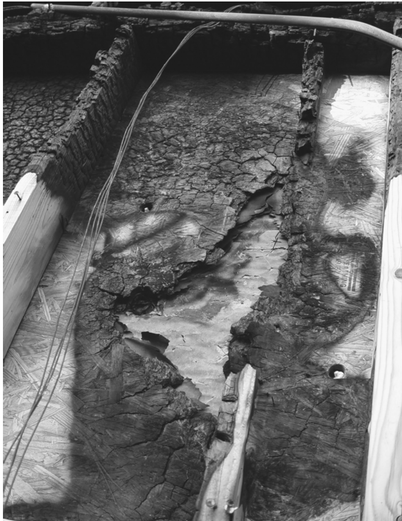
Figure 2 - Stucco scorching inside at point of origin
